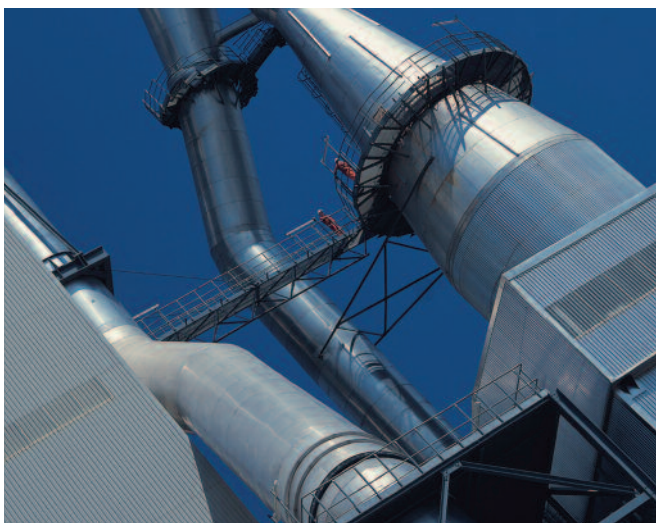
The concrete industry has invested in plant to improve environmental performance. For example in the cement sector the majority of dust from the kiln is collected and recycled.
